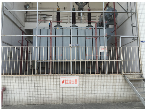
110kV 永康站现有站内主变
