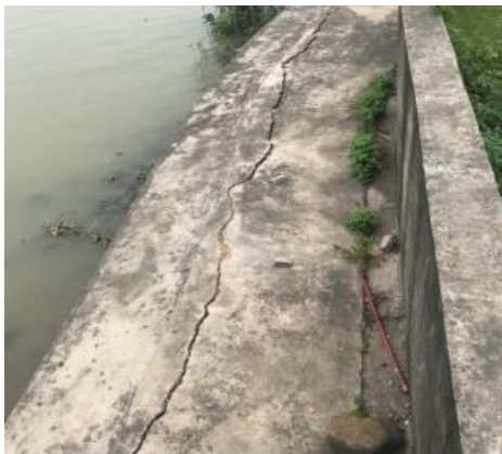
砼面板沉降引起纵向裂缝
